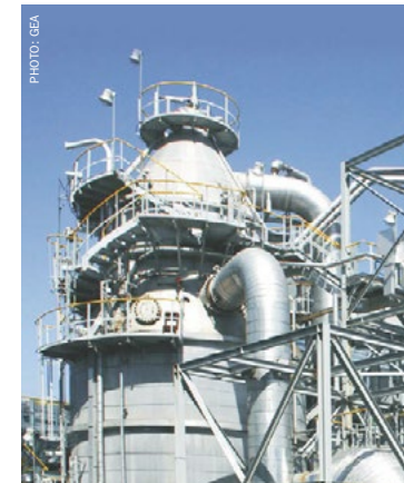
Operational GEA crystalliser at a fertilizer production plant.
