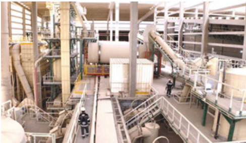
OCP’s TSP Hub at Jorf Lasfar is an industrial programme designed to support changing agricultural practices and address diverse fertilization needs.
