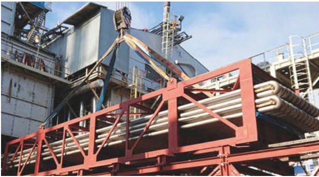
Fig. 4: One-shot pull-in revamp solution for mixed feed coil.
