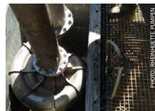
The vertical pump is installed in the tank of the sulphuric acid plant.
