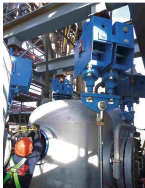
Fig. 10: 1102-C hanging on spring supports.
