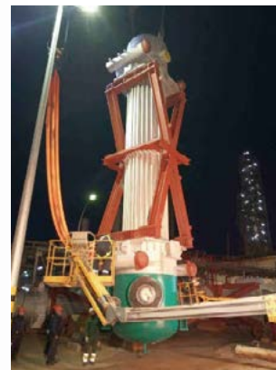
Fig. 3: Item 1101-C positioned vertically.
