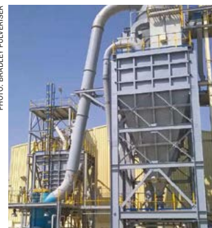
PHOTO: BRADLEY PULVERISER Air-swept mill system.
