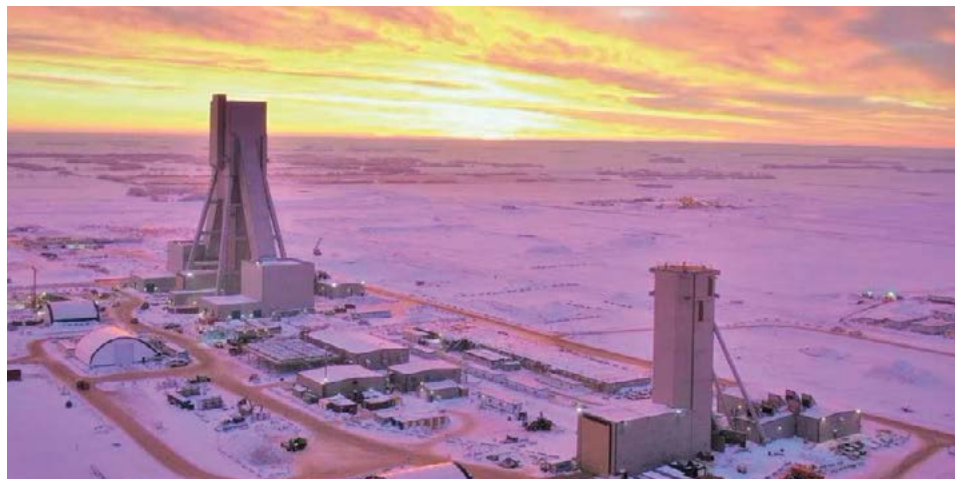
The 4.35 million t/a capacity Jansen S1 project is expected to produce its first potash ore towards the end of 2026, following a six-year construction phase. The project is located 140 kilometres east of Saskatoon, Saskatchewan.
