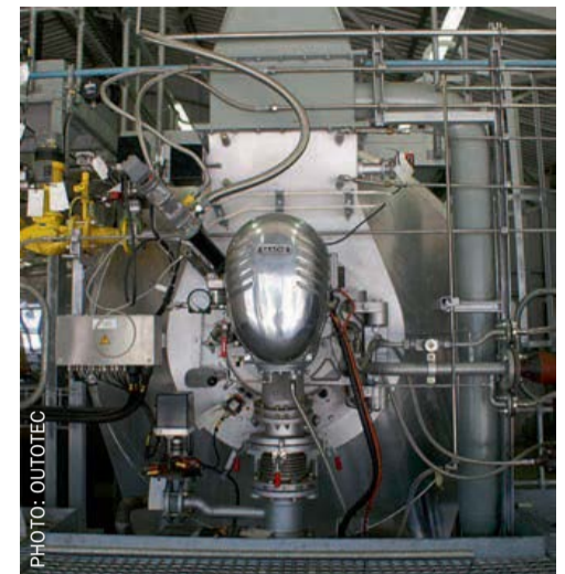
Fig. 8: View of the LURO burner on the combustion module.
