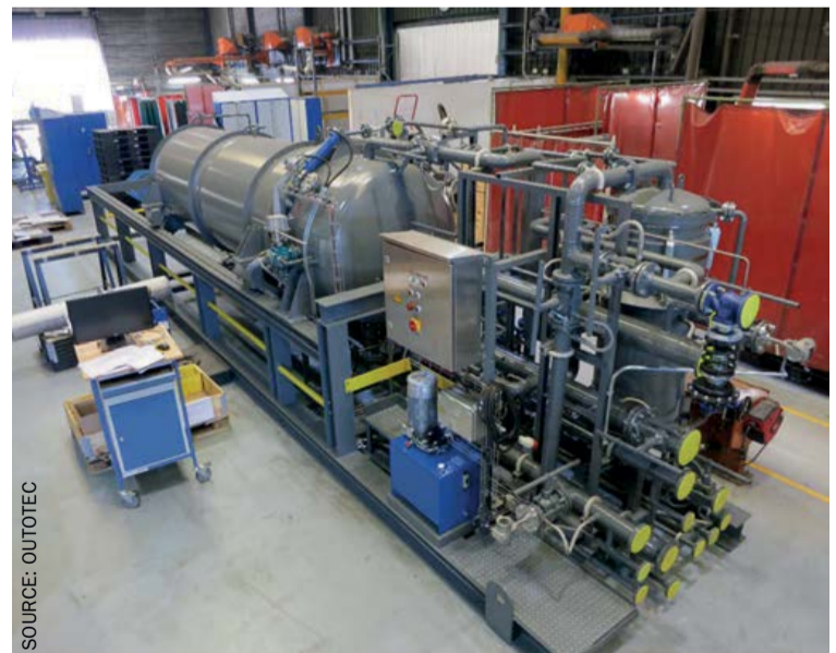
Fig. 6: Sulphur filtration module at workshop.
