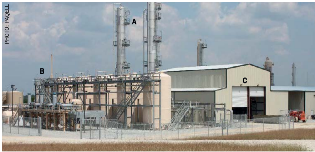
Fig. 2: Treating facility, showing the absorbers (A), bioreactors (B) and sulphur recovery building (C).
