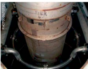
Fig. 10: Acid distribution in the packed bed stage of the venturi absorption towers.
