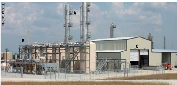
Fig. 2: Treating facility, showing the absorbers (A), bioreactors (B) and sulphur recovery building (C).
