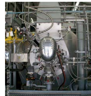
Fig. 8: View of the LUR0 burner on the combustion module.
