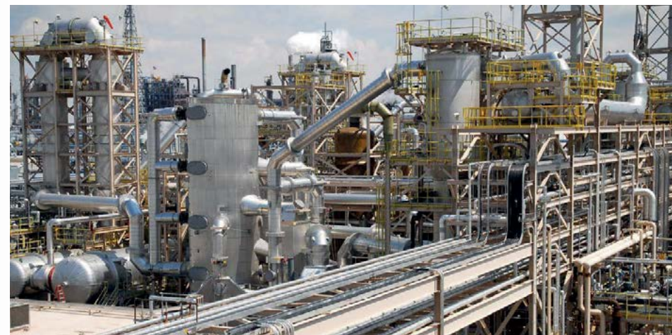
MECS® ZeCor® is used throughout the sulphuric acid plant.
