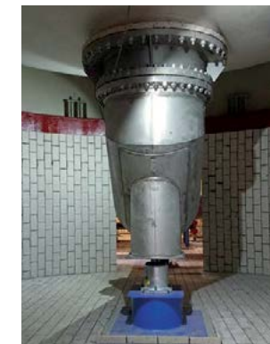
Acid piping fabricated in NORAM SX™ alloy.
