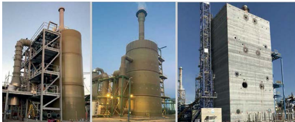
Examples of Sulfacid® industrial installations.
