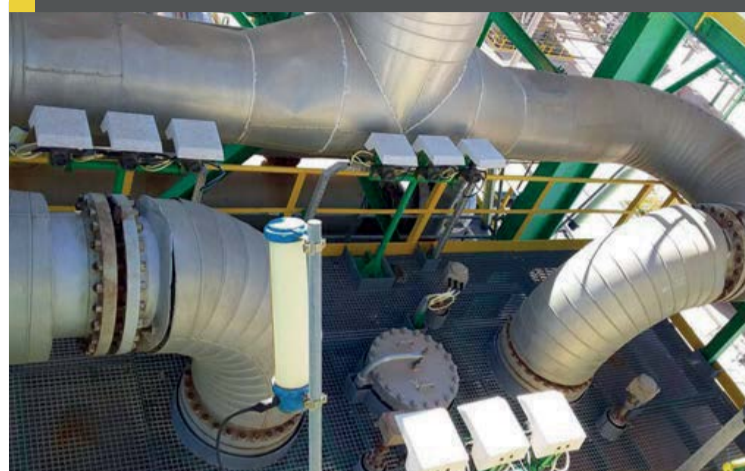
Fig. 9: Reducing reactor top manhole
