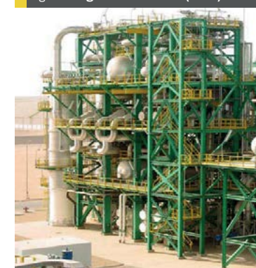
Fig. 3: Tail gas treatment unit (TGTU)
