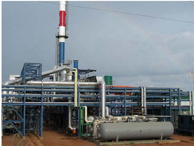
Sulphuric acid plant with integrated liquid SO 2 production.
