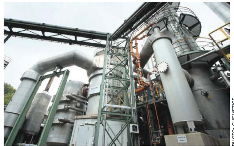
Fig. 4: CORE™ add-on system in operation.
