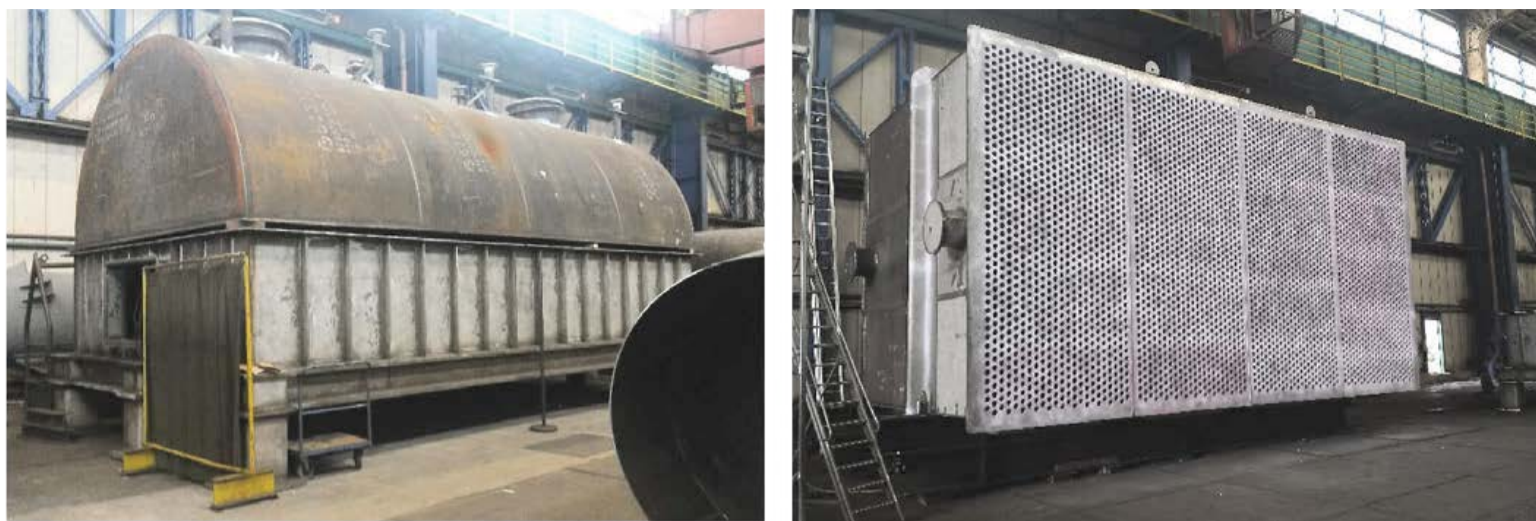
Fig. 6: CORE™ reactor under construction: top and bottom vestibules (left), central tube section (right)
