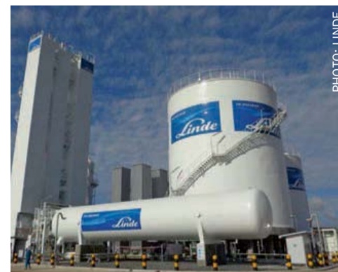
Cryogenic air separation plant.
