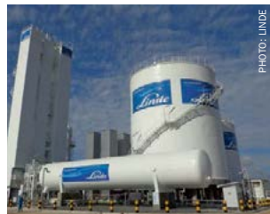
Cryogenic air separation plant.
