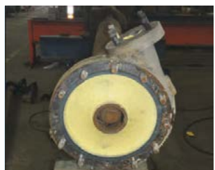
Fig. 9: Lewis® sulphur pump after removal from service, showing a heavy layer of sulphur under the suction head.
