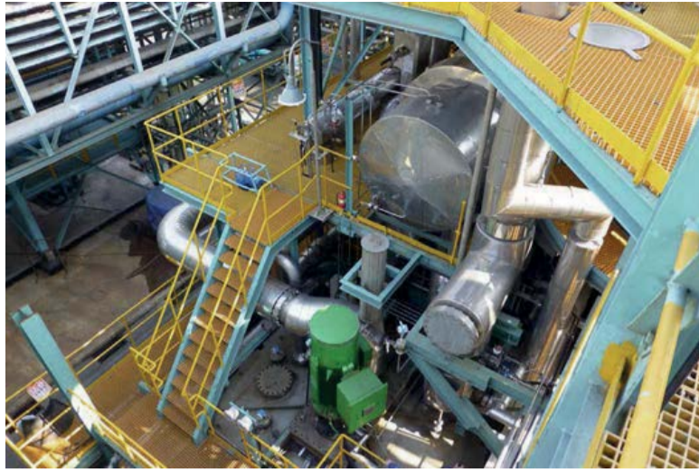
Left: Installed Outotec HEROS™ system.
