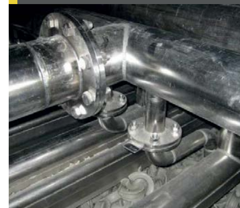
Fig. 4: Dual operation FIDI™ system installed
