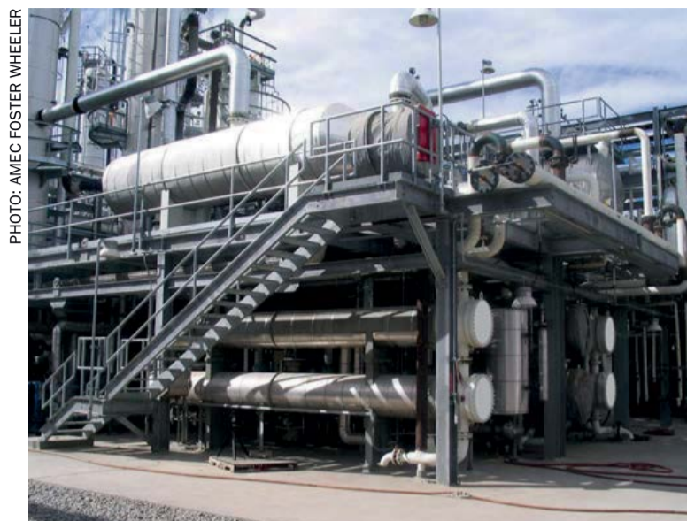
Fig. 2: View of modular installation, note lower module structure is covered by finished concrete.
