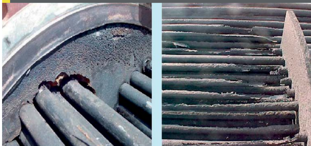
Fig 13: Reboilers corroded by excessive acid gas breakout
