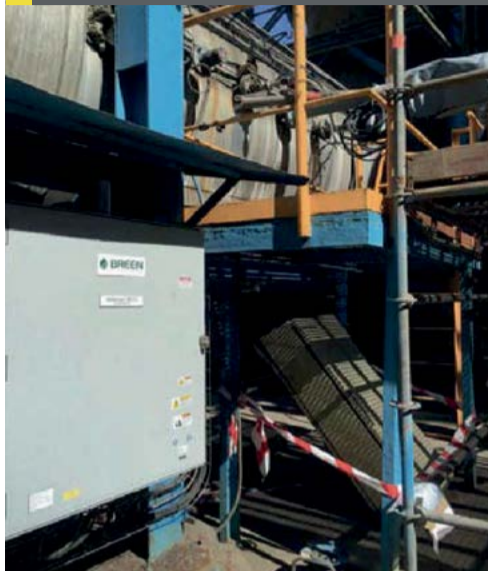
Fig 4: System installation at Atlantic Copper, Huelva, Spain
