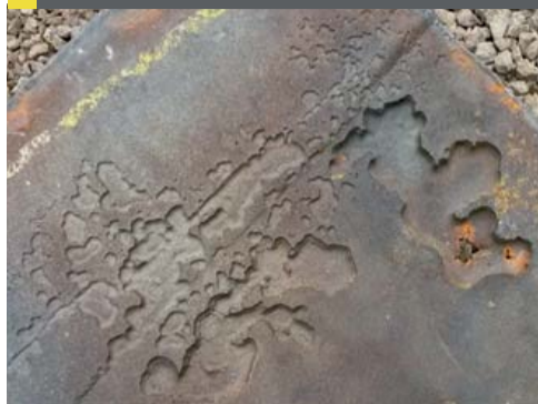
Fig 14: Severe acid attack in regenerator bottom section
