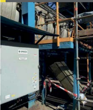
Fig 4: System installation at Atlantic Copper, Huelva, Spain
