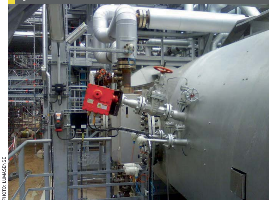
Fig 3: Lumasense Pulsar 4 installation
