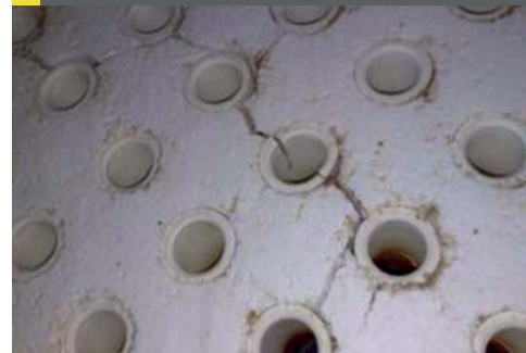
Fig 8: Cracks in tube sheet refractory
