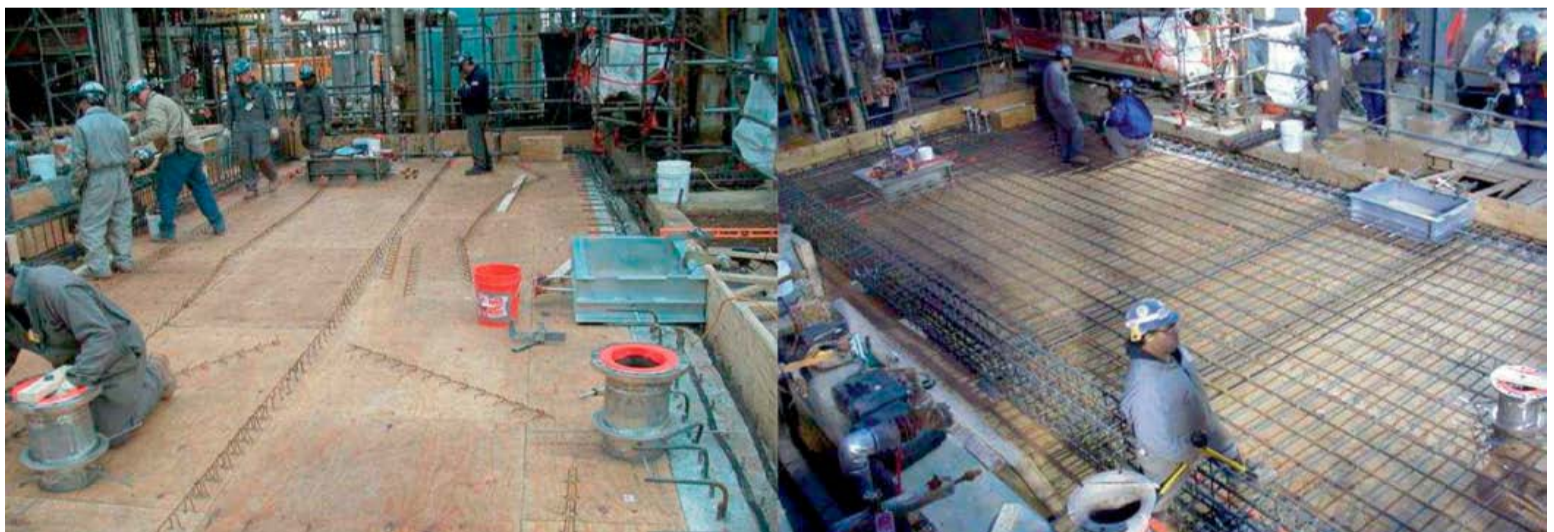
Fig. 5: Sleeved process piping penetrations and entry portals positioned prior to sulphur pit roof slab concrete placement.
