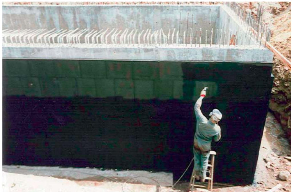
Fig. 8: View of a spray applied waterproofing membrane placed on top of insulating board adhered to the external concrete surface of a new sulphur pit.
