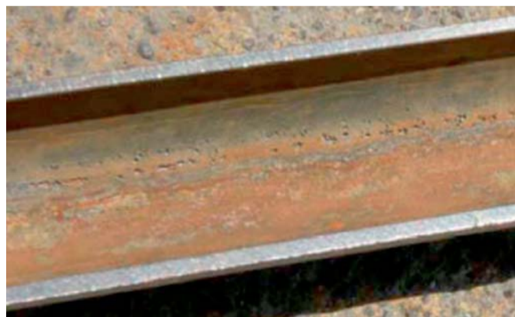
Fig. 3: Chloride pitting in bore of extracted tube.
