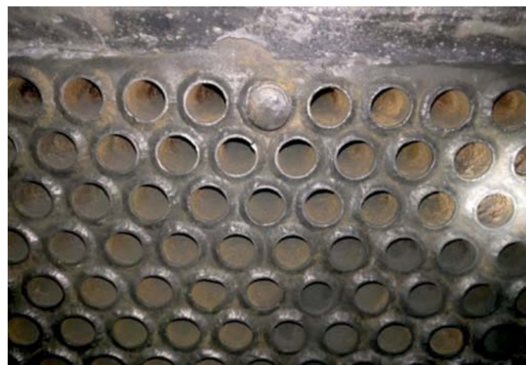
Fig. 2: Aluminised tube sheet after cleaning.
