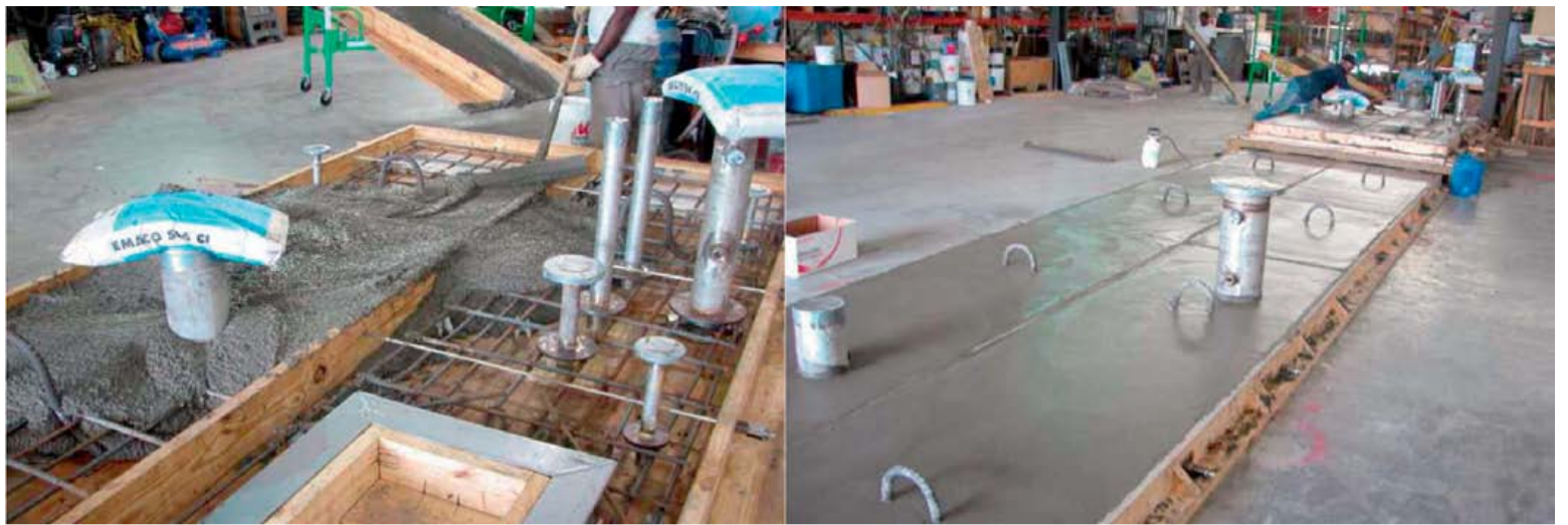
Fig. 6: Precast concrete sulphur pit roof slab panels that incorporate “spool” penetrations installed during concrete casting/placement.
