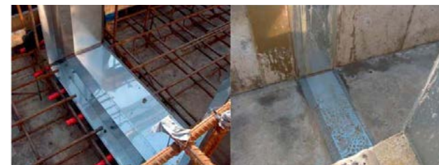
Fig. 2: Stainless steel expansion joint detail along the side walls and floor of a sulphur trench.
