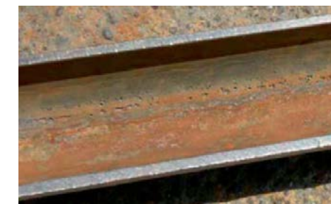
Fig. 3: Chloride pitting in bore of extracted tube.
