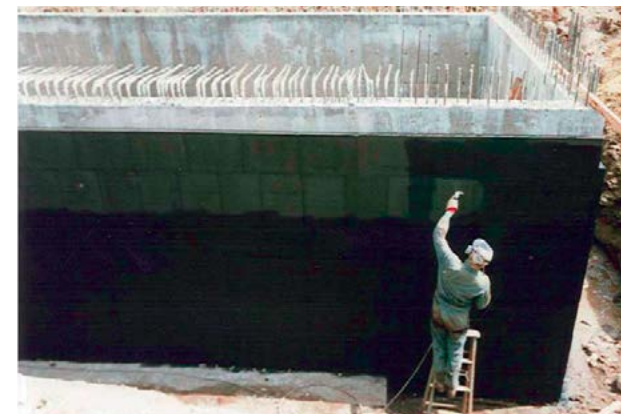
Fig. 8: View of a spray applied waterproofing membrane placed on top of insulating board adhered to the external concrete surface of a new sulphur pit.
