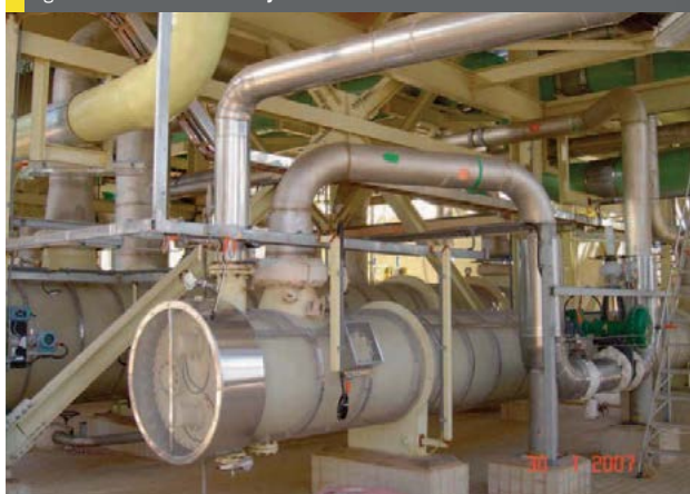
Fig 4: Hot water heat recovery acid coolers
