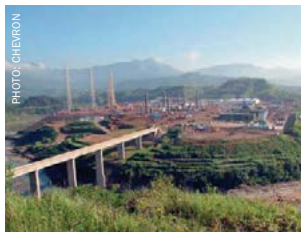
Luojiazhai gas plant.
