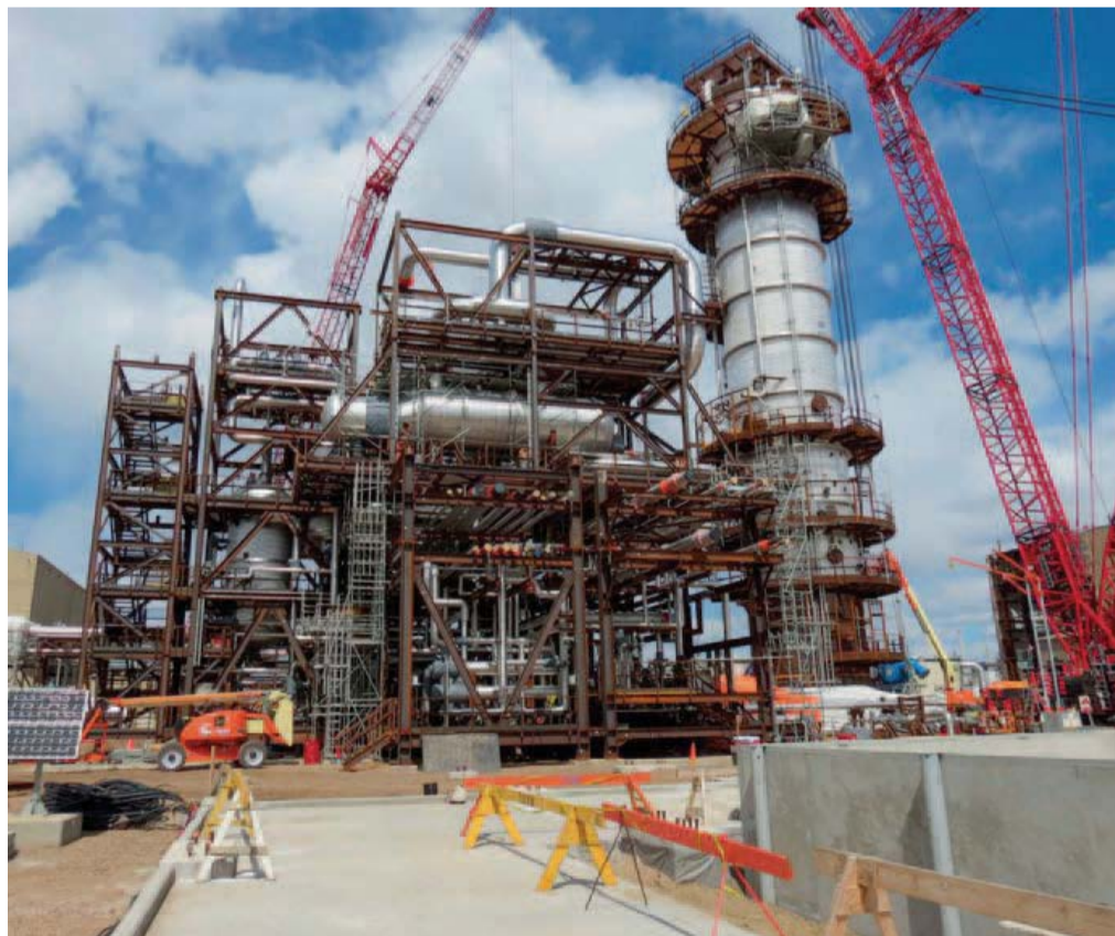
The CCS project at Shell's Scotford Upgrader, Alberta.
