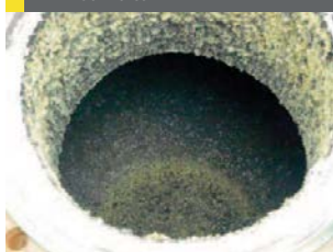
Fig 4: Compact material found on the top of the catalyst of the first converter
