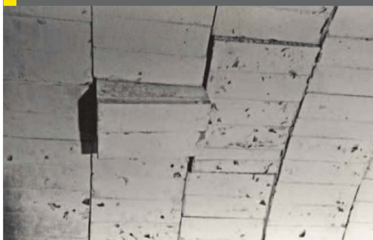
Fig 5: Brick slippage due to insufficient keying action
