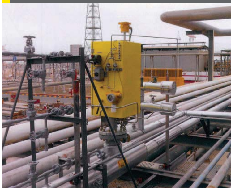
Fig 8: Sample probe cabinet site installation
