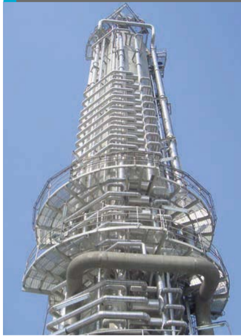
Fig. 24: Nitric acid absorption tower
