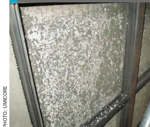
Fig. 7: Insulation blinding the catalyst surface
