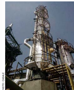
Fig. 1: New process condensate stripper
