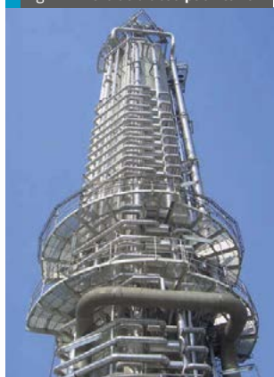
Fig. 24: Nitric acid absorption tower
