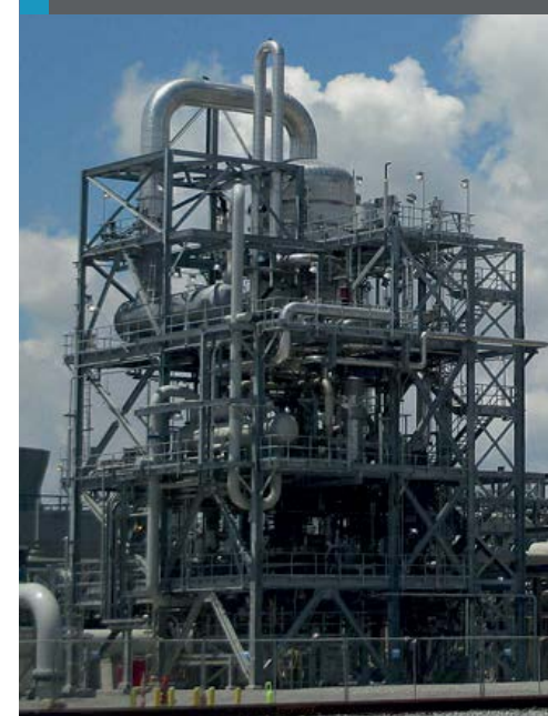
Fig. 3: Mega UAN plant at CFI in Donaldsonville, USA
