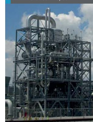
Fig. 3: Mega UAN plant at CFI in Donaldsonville, USA
