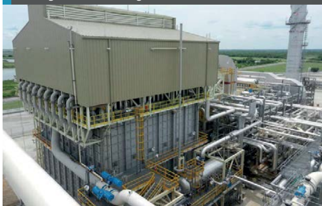
Fig. 1: Top-fired tkIS Uhde steam reformer with the PSA offgas line and the offgas manifold in the foreground
