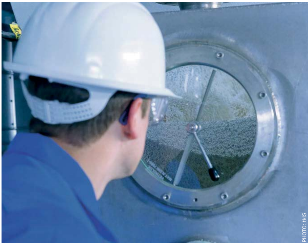
Fig. 4: The fluidised bed granulator is the centrepiece of the production plant.
