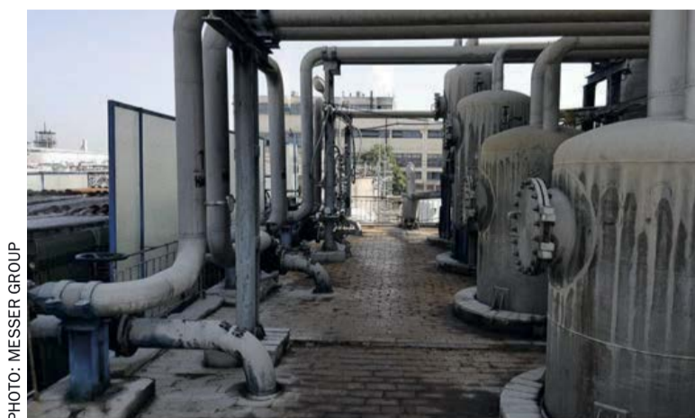
Fig. 4: Heat exchangers (left) and buffer vessels for the pumps (right) which are filled with weak acid from the absorption process from nitric acid Line II.
