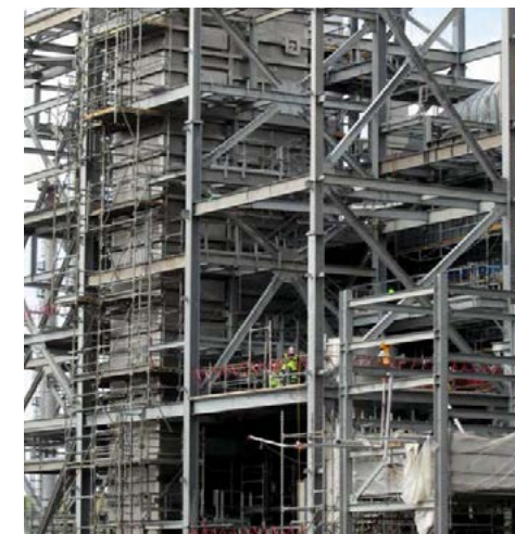
Fig. 8: Construction phase of a rectangular modularized MMV scrubber installation for a 1,000 t/d urea granulator.
