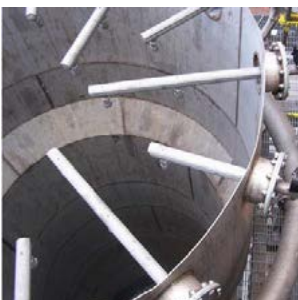
Fig. 3: View of a typical SpiralMist quench stage.
