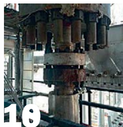
16 Plant Manager+ Leak in a high pressure connection to the urea reactor.
