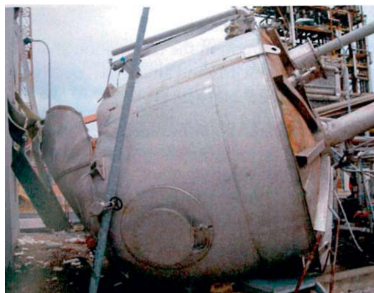
Fig. 10: Ruptured aqueous ammonia storage tank, Europe, 2009.
