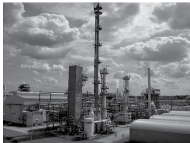
13,200 Nm³/hr Hydrogen Plant
