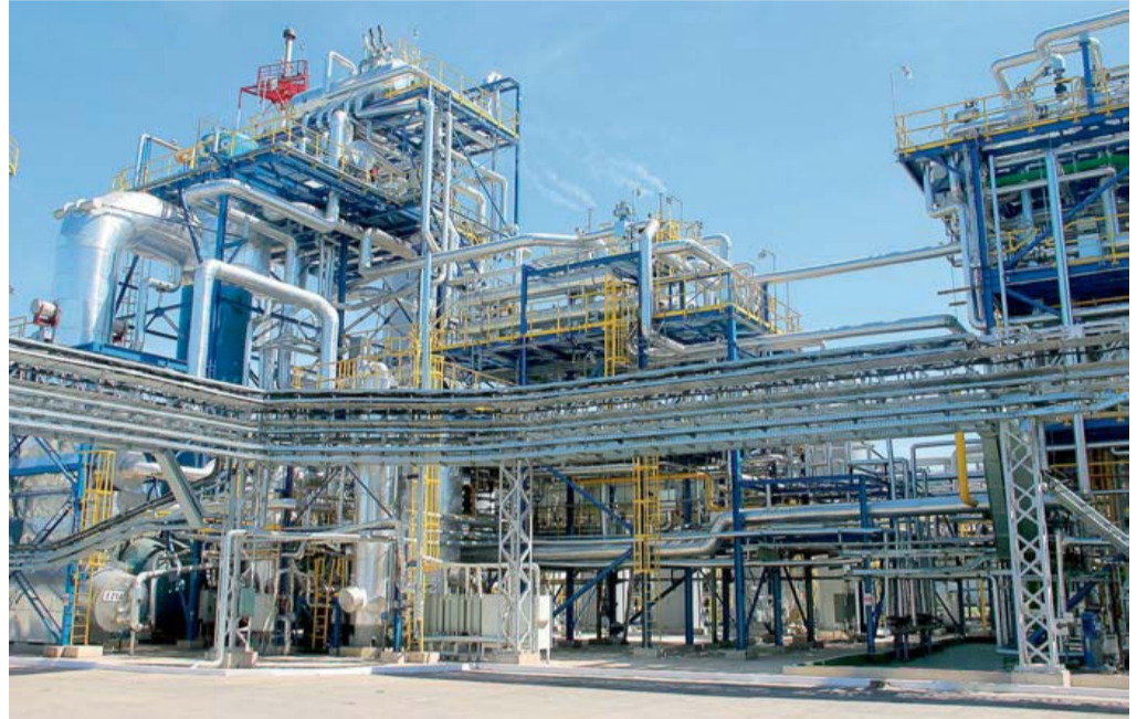
Shchekinoazot 's existing methanol facility.
