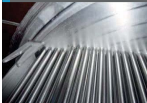
Fig 9: Excellent condition of tubes in pool condenser
