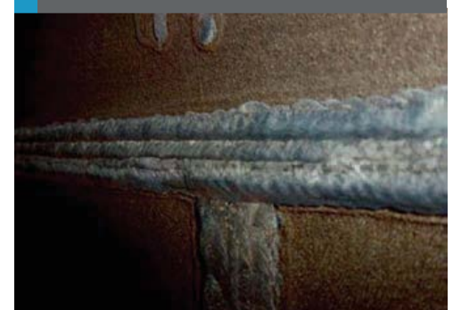
Fig 4: Lining and welding seams of reactor
