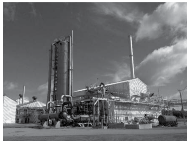
500 TPD Nitric Acid Plant, Weatherly
