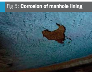
Fig 5: Corrosion of manhole lining
