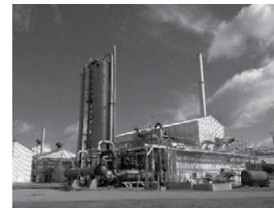
500 TPD Nitric Acid Plant, Weatherly
