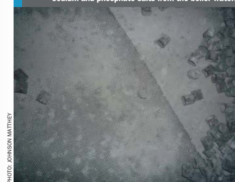
Fig 13: Top of a HTS catalyst bed grid badly clogged with sodium and phosphate salts from the boiler water.
