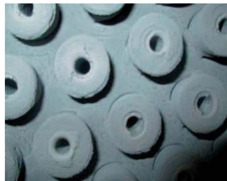
Blocked orifice plugs in circulation heater bottom and top liquid divider blockage.
