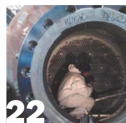
22 Corrosion in urea plants Mitigating the effects of carbamate corrosion.
