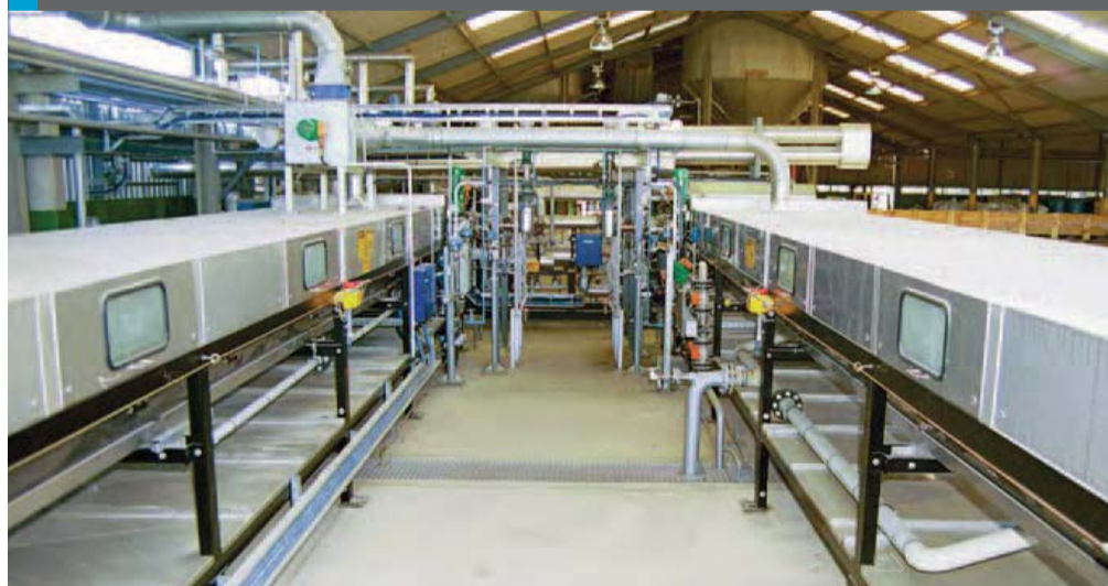
Fig 6: Rotoform skid-mounted equipment showing hood
