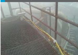
Fig 10: NH 3 monitoring at top of prilling tower with 2m open path measurement. Note persistent mist
