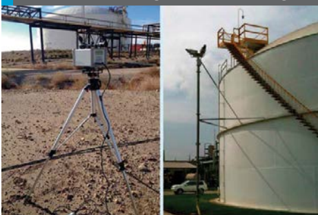
Fig 8: Ammonia storage tank monitoring. Temporary monitoring with GasFinder2 on left. Permanent monitoring with GasFinderMC on right
