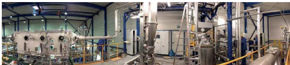
Thiogro Urea-ES installation at tkFT pilot plant in Dortmund Germany.
