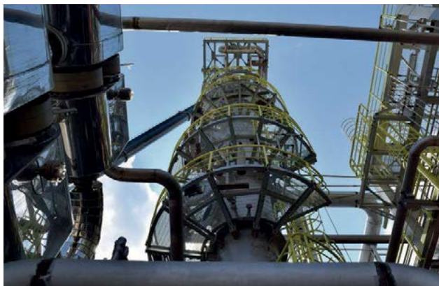
The new EuroChem Northwest world-scale ammonia plant near St Petersburg.
