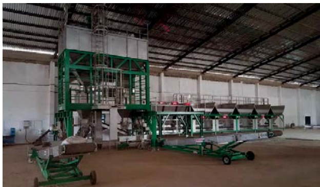
EMT Weighcont blender and bagging machine at a fertilizer blending factory in Ghana.
