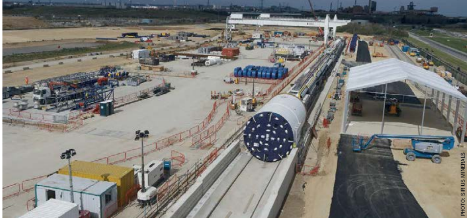
The first tunnel boring machine Stella Rose at entrance of Teesside tunnel.
