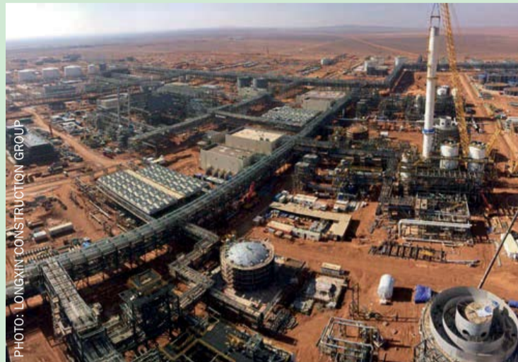
Ma'aden Wa'ad Al-Shamal Phosphate Company's Umm Wu'al mega project was completed in August 2017.
