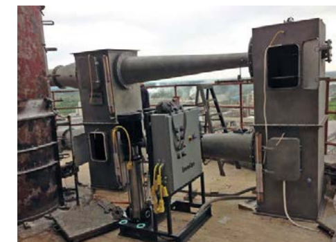
Fig. 9: Pilot Jet Scrubber located on top of prilling tower for emissions testing.
