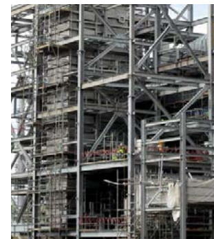
Fig. 7: Construction phase of a rectangular modular MMV scrubber installation for a 1,000 t/d urea granulator.
